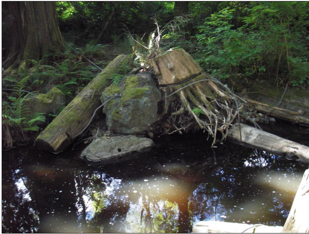
FIGURE 18.51 Large rocks and cables can be used to anchor large woody debris placed in channels for habitat improvement. (Site work by W. Pollard; photo: G. Horel)
