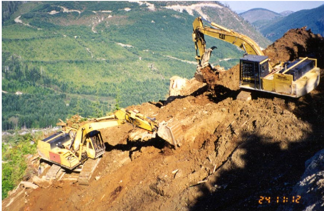
FIGURE 18.18 Two excavators using a double-bench approach to deactivate a road with deep fills on south-central Vancouver Island. The lower machine passes material to the upper machine, which places it against the cutslope. (Photo: D. Ostapowich)
