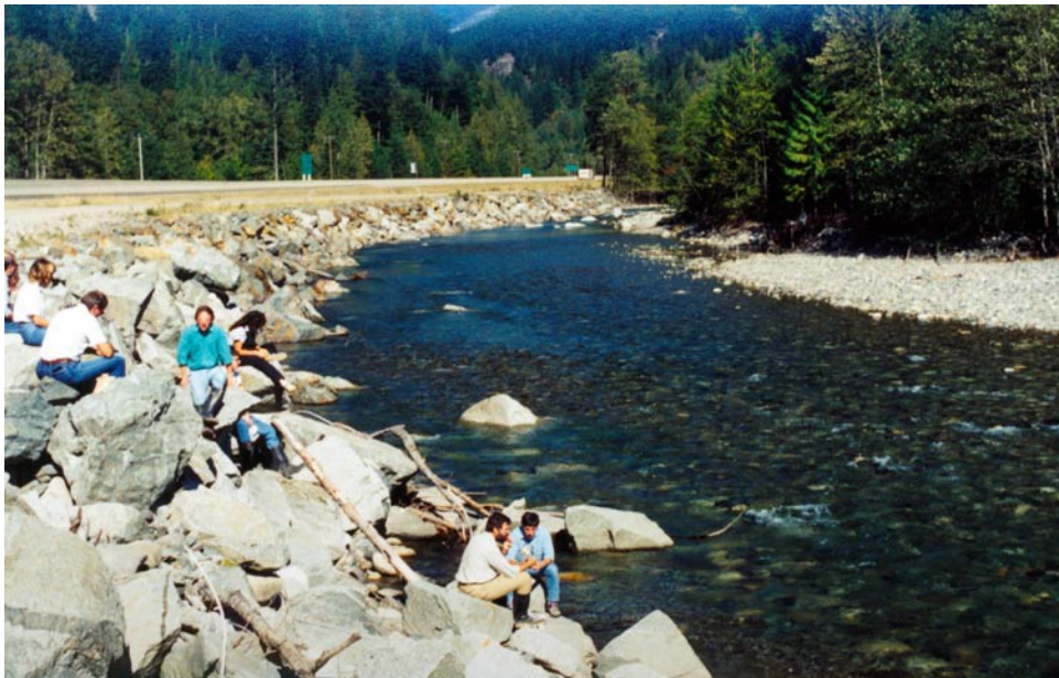
FIGURE 18.43 Coquihalla River, 1991: Local scour associated with flood flows caused the boulders to sink and become buried in the channel bed. (Photo: M. Miles)
