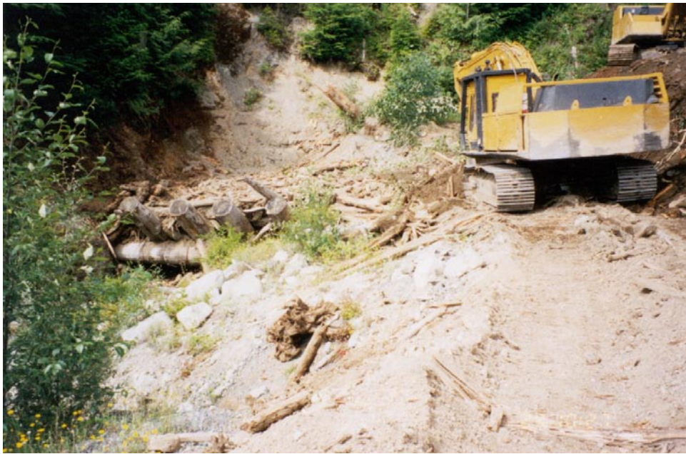
FIGURE 18.14 Debris rack upstream of culvert on unmaintained road. Debris rack had completely filled in and was starting to collapse. (Photo: D. Ostapowich)
