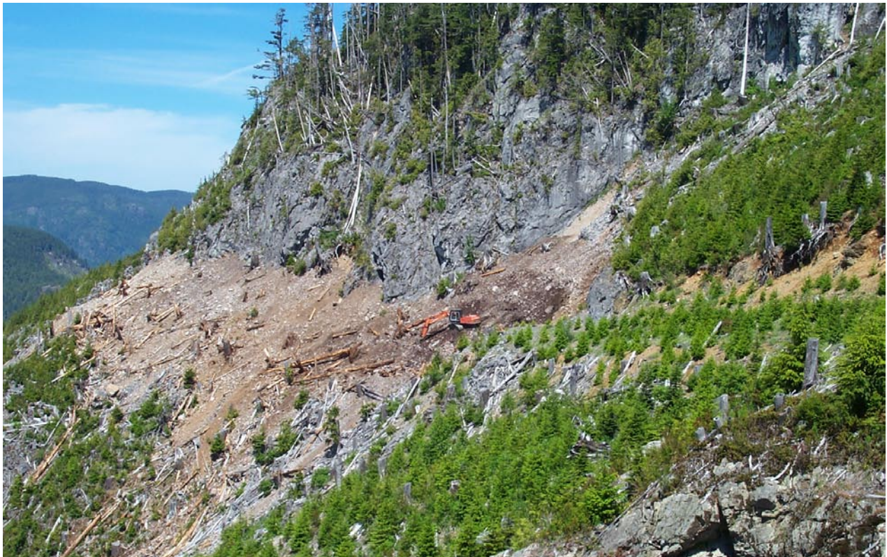
FIGURE 18.21 This road section is undergoing full deconstruction by retrieving sidecast fill material and placing it against the cut, removing drainage structures, and placing salvaged wood on the regraded slope. (Photo: D. Ostapowich)
