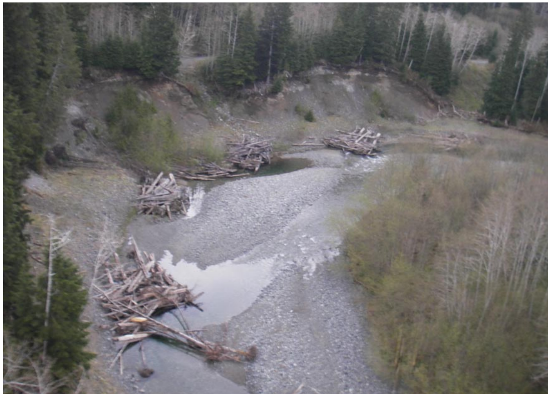
FIGURE 18.48 A series of engineered logjams placed to reduce flow velocities at the base of the embankment allows vegetation to become established on the slopes. (Design by M. Sheng; site supervision by M. Wright; photo: G. Horel)
