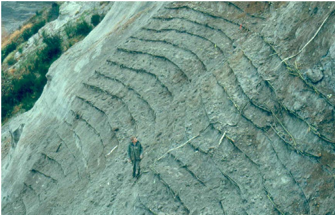
FIGURE 18.23 Wattle fences can be used to treat steep slopes where surface raveling is preventing plant growth. (Photo: D. Polster)
