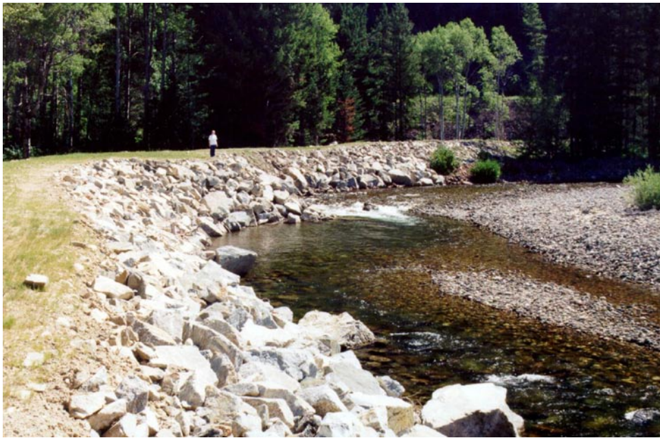
FIGURE 18.44 Hydraulically rough riprap formed of large rock and short spurs can be used to enhance fisheries habitat values along short sections of the riprap. (Photo: M. Miles)
