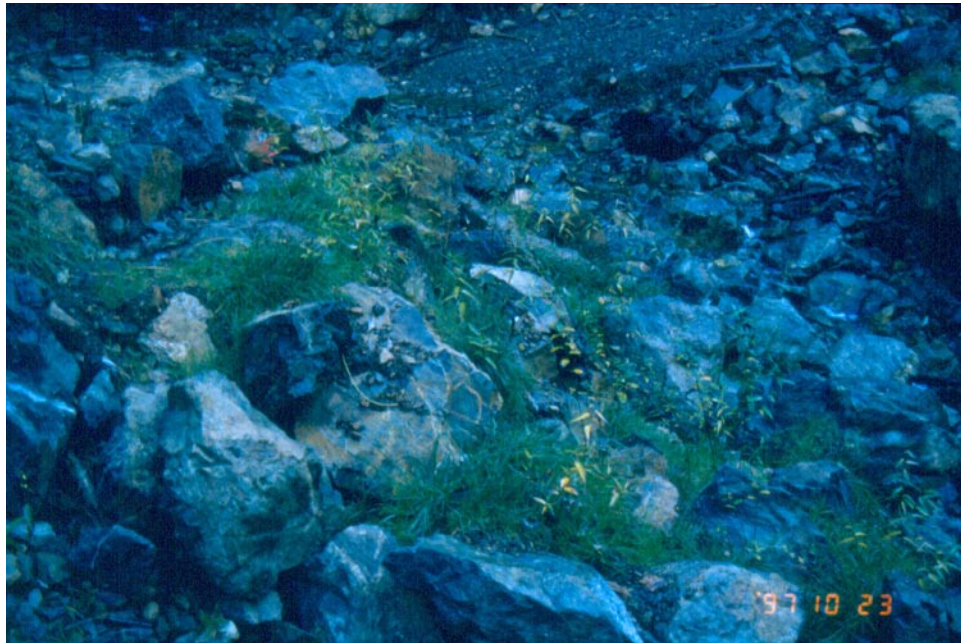
FIGURE 18.20 The culvert was removed at this crossing and the drainage course restored with an armoured swale. Pocket planting was used to establish vegetation in the riprap. (Photo: D. Polster)
