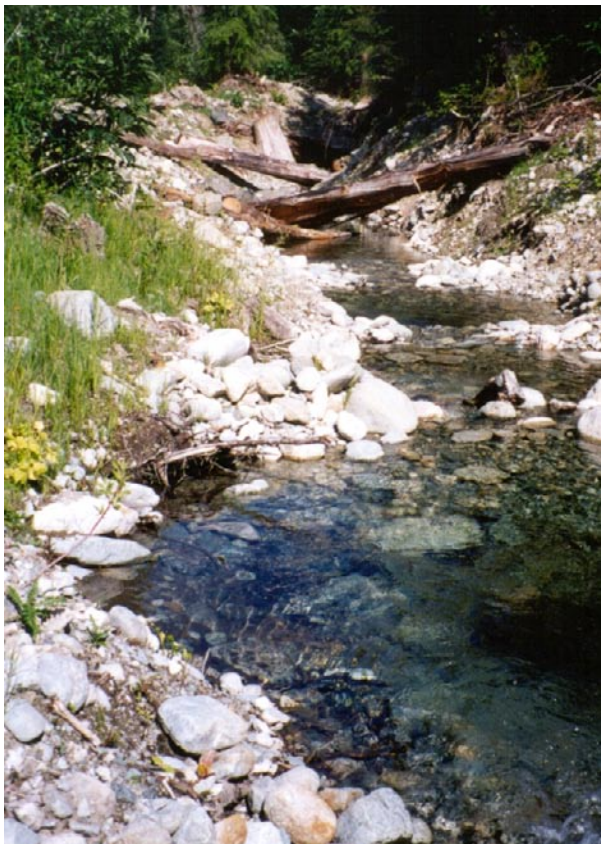
FIGURE 18.55 Channel excavated to connect gravel pit to Taylor River. (Site work by M. Wright; photo: G. Horel)
