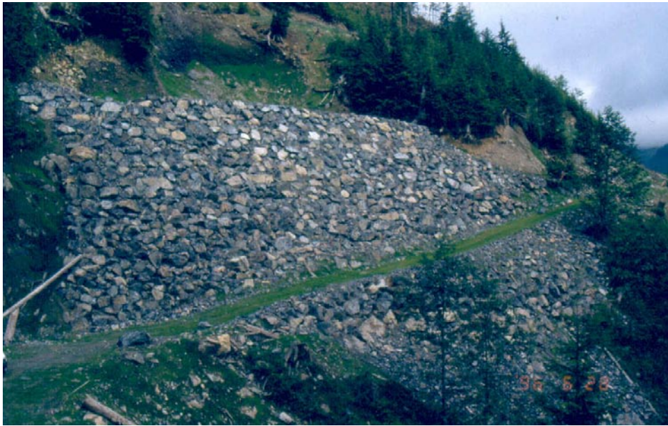
FIGURE 18.10 A retaining basin was constructed to capture materials that will fall from the slope above. (Photo: D. Polster)
