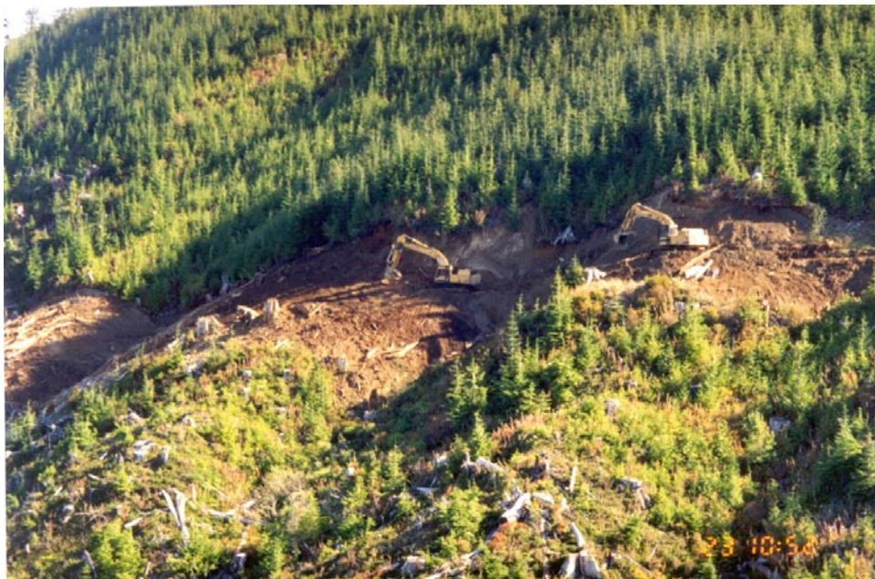
FIGURE 18.17 Permanent deactivation and hillslope contouring on a road in south-central Vancouver Island. (Photo: D. Ostapowich)
