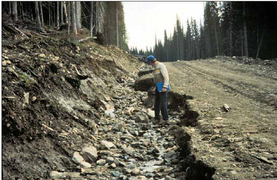
FIGURE 9.25 Insufficient cross-drainage resulted in the capture and routing of water along road ditches. (Photo: J. Schwab)
