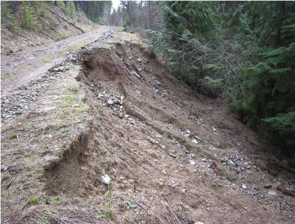
FIGURE 9.11 Road-fill failure in the Kid Creek area of the Kootenay Lake Forest District, 2007; failure was caused by drainage diversion that saturated the road fill. (Photo: P. Jordan)
