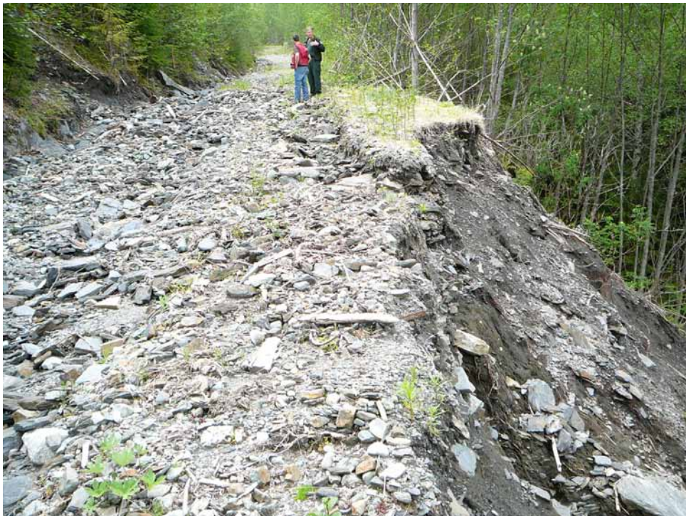
FIGURE 9.17 Road surface and slide headscarp from Figure 9.16. Note heavily eroded road surface. Several blocked culverts led to large volumes of water flowing onto the fillslope at the headscarp of both slides. (Photo: T. Millard)
