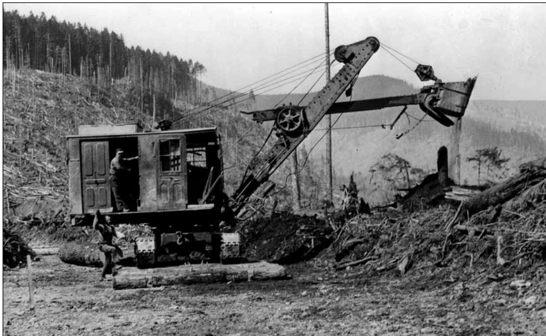
FIGURE 5.10 Road construction with a line shovel in 1936. (Photo: Royal BC Museum Archives, NA-06671)
