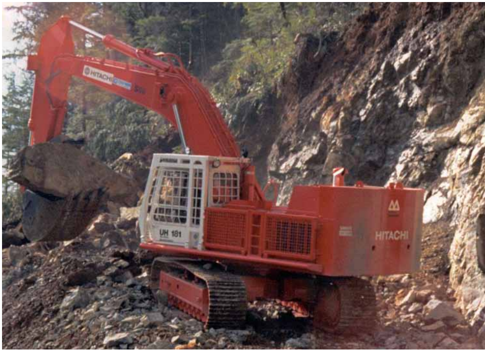
FIGURE 5.13 The hydraulic excavator brought significant change to the quality of constructed roads. (Photo: D. Bendickson)
