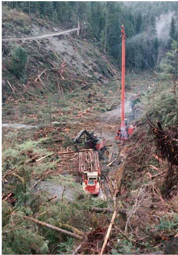
FIGURE 1.2 Logging on the Carnation Creek floodplain, 1976. (Photo: Natural Resources Canada, Canadian Forest Service)
