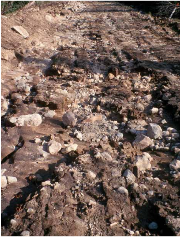
FIGURE 9.29 Surface erosion on a road near Redfish Creek in the Kootenay Lake Forest District in 1993, caused by a plugged culvert and inadequate water bars. (Photo: P. Jordan)
