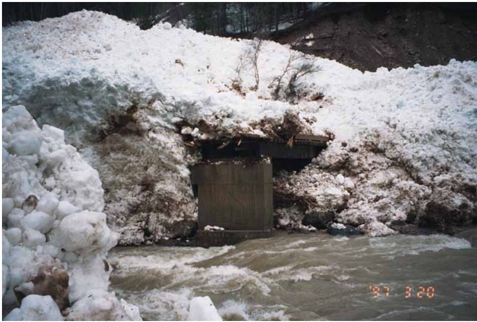
FIGURE 9.45 Close-up of the destroyed bridge on Bull River (see Figure 9.44 above). (Photo: D. Toews)
