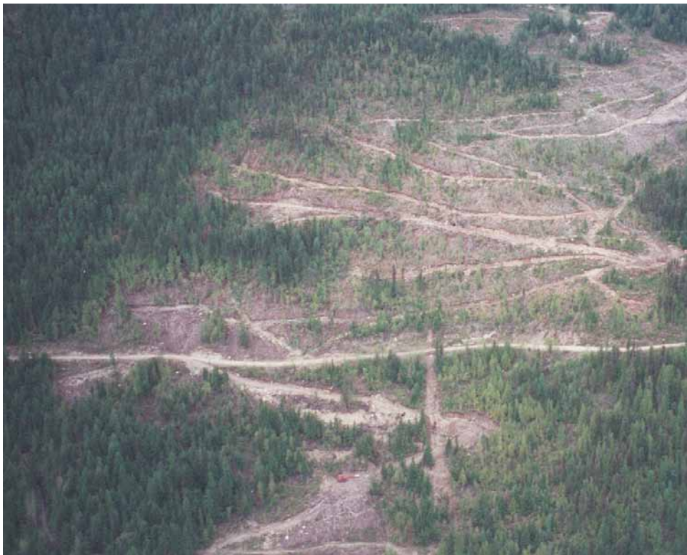
FIGURE 9.15 Debris slide/avalanche that involved a fill failure of a mainline Forest Service road near Giveout Creek in the Kootenay Lake Forest District, 2002. The debris slide was caused by drainage diversion on skid trails on private land above. Although ground-based logging of steep slopes is no longer practised on Crown land, it still sometimes occurs on private land. (Photo: P. Jordan)
